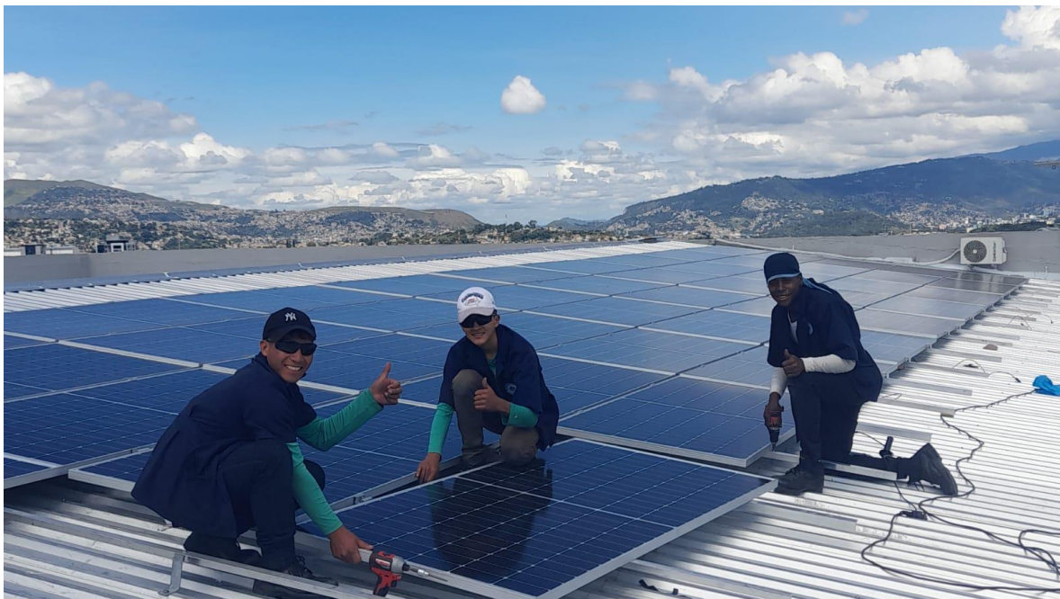
Learning to install solar panels – On the Job Work Immersion for our Boystown students – November 2022
