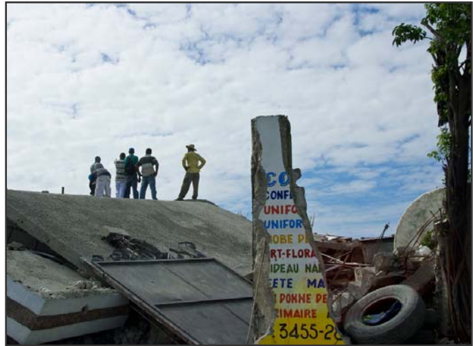
A group of men atop a collapsed building in Port-au-Prince. Save the Children photo.
